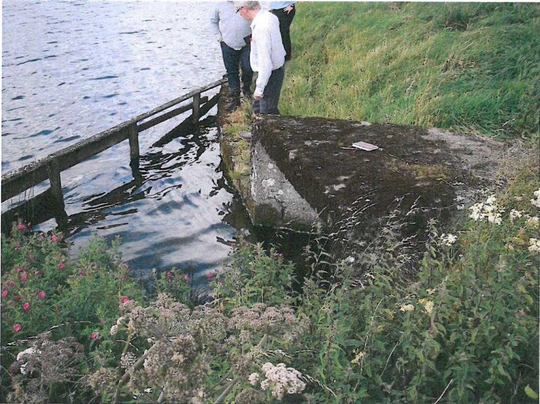
Photo 6 – Spillway inlet showing damaged baffle board
